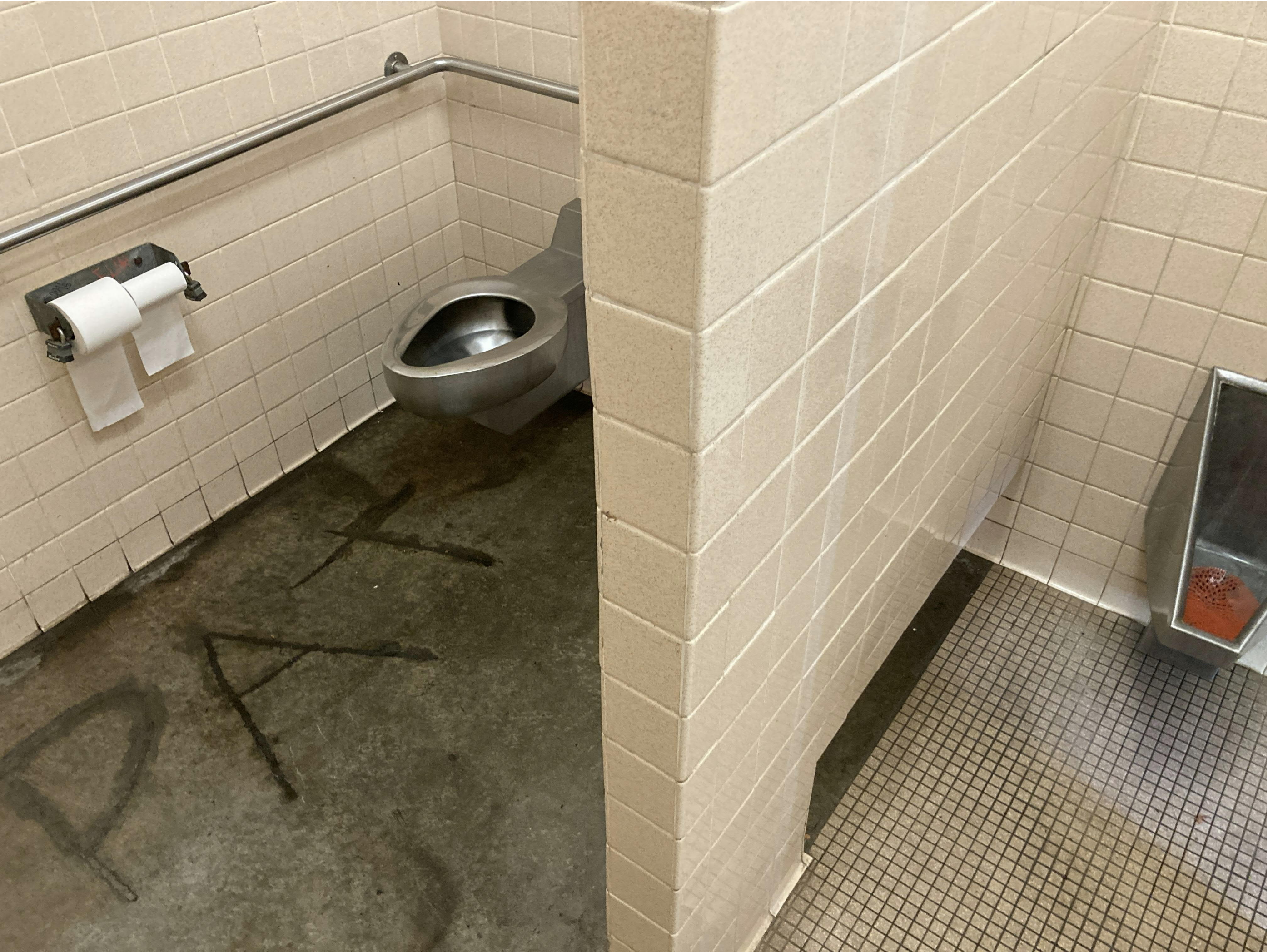
PUBLIC RESTROOM ARE OLD, VANDALIZED, AND LACK PRIVACY
