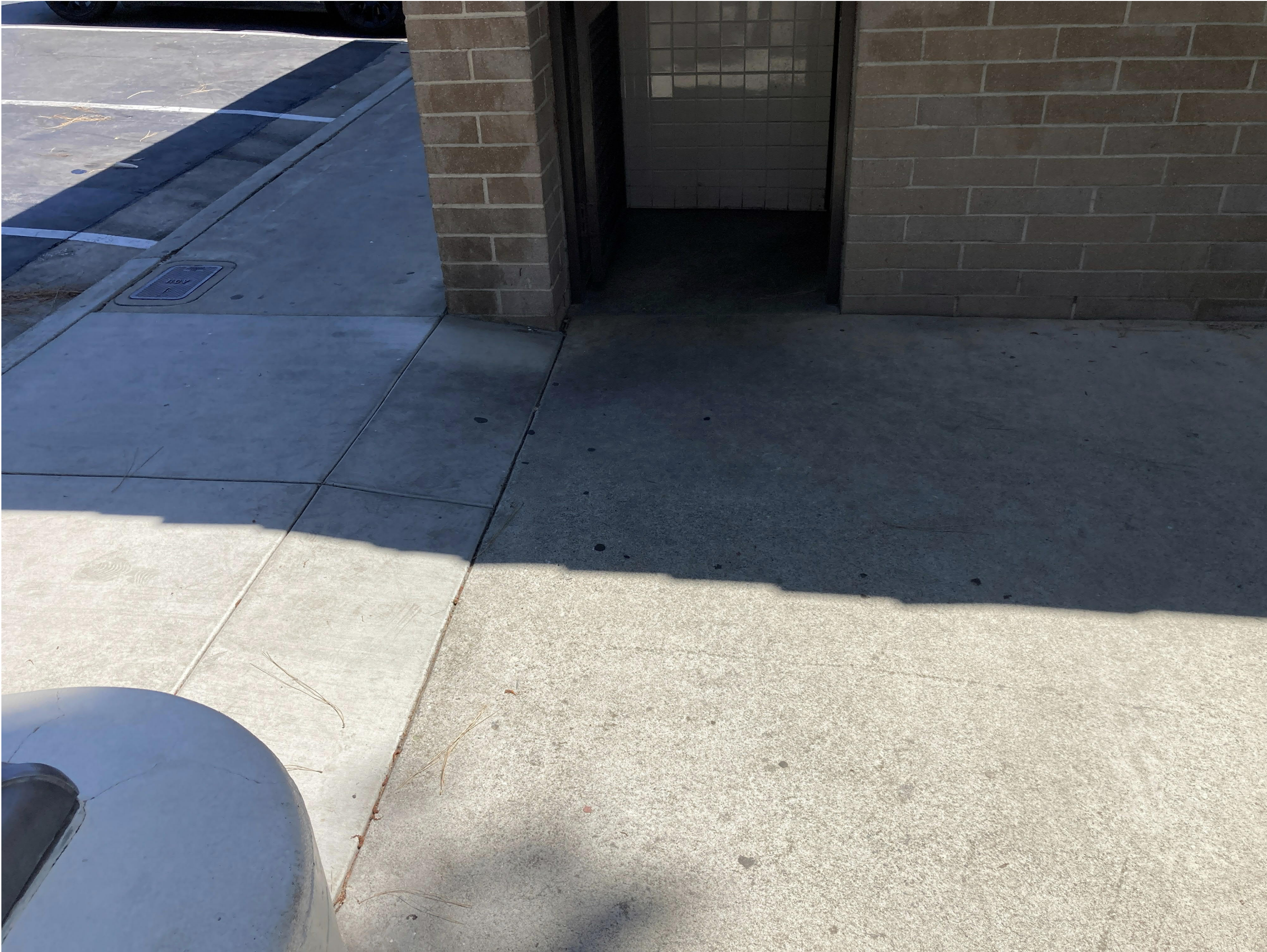
UNEVEN LANDING OUT SIDE OF RESTROOM
