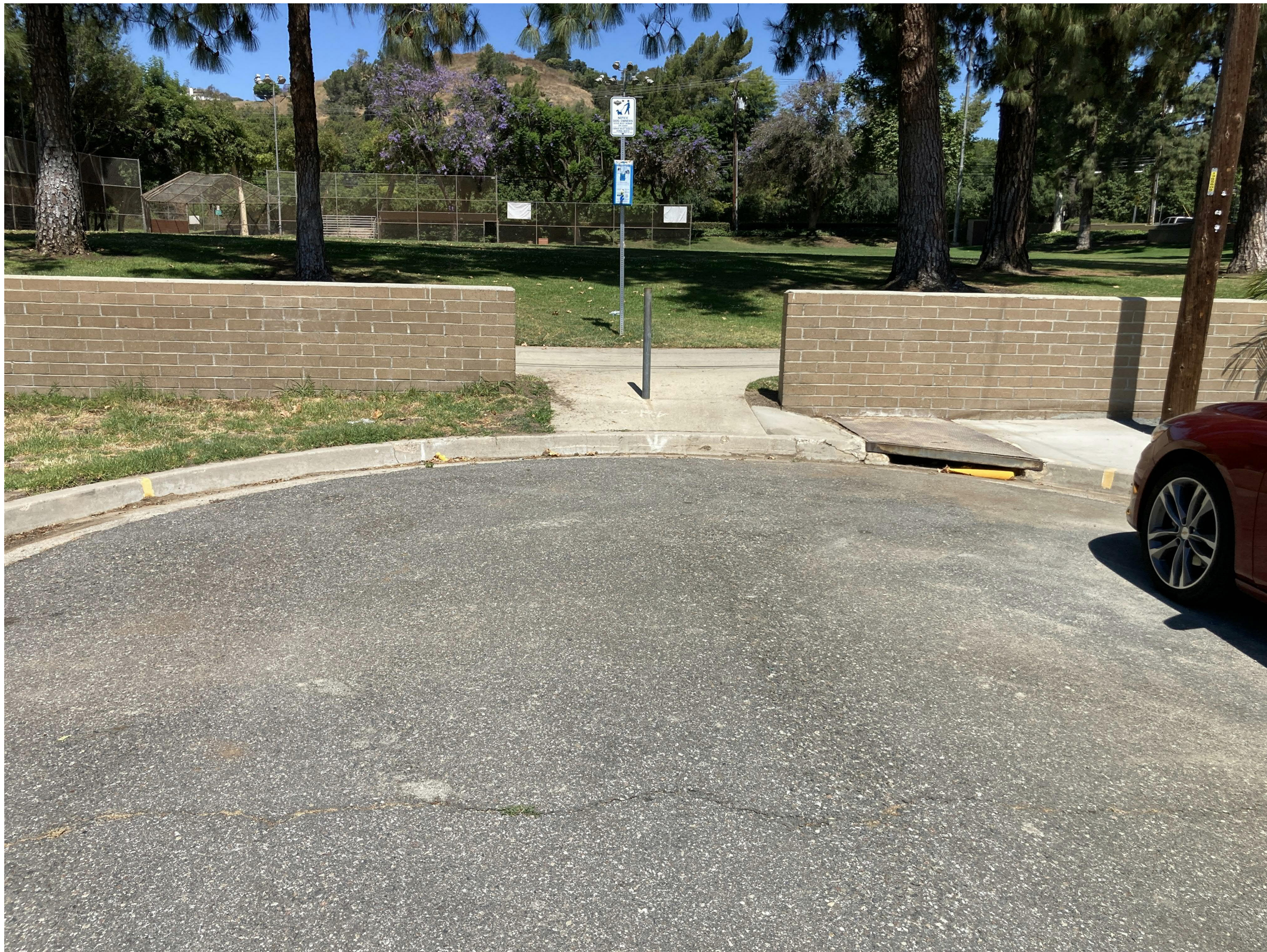
SOUTH PARK ENTRANCE LACK DISTINCTION AND ADA ACCESS
