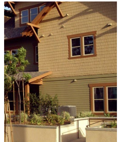
Figure 6-28 - Painted Shingles Over Siding
